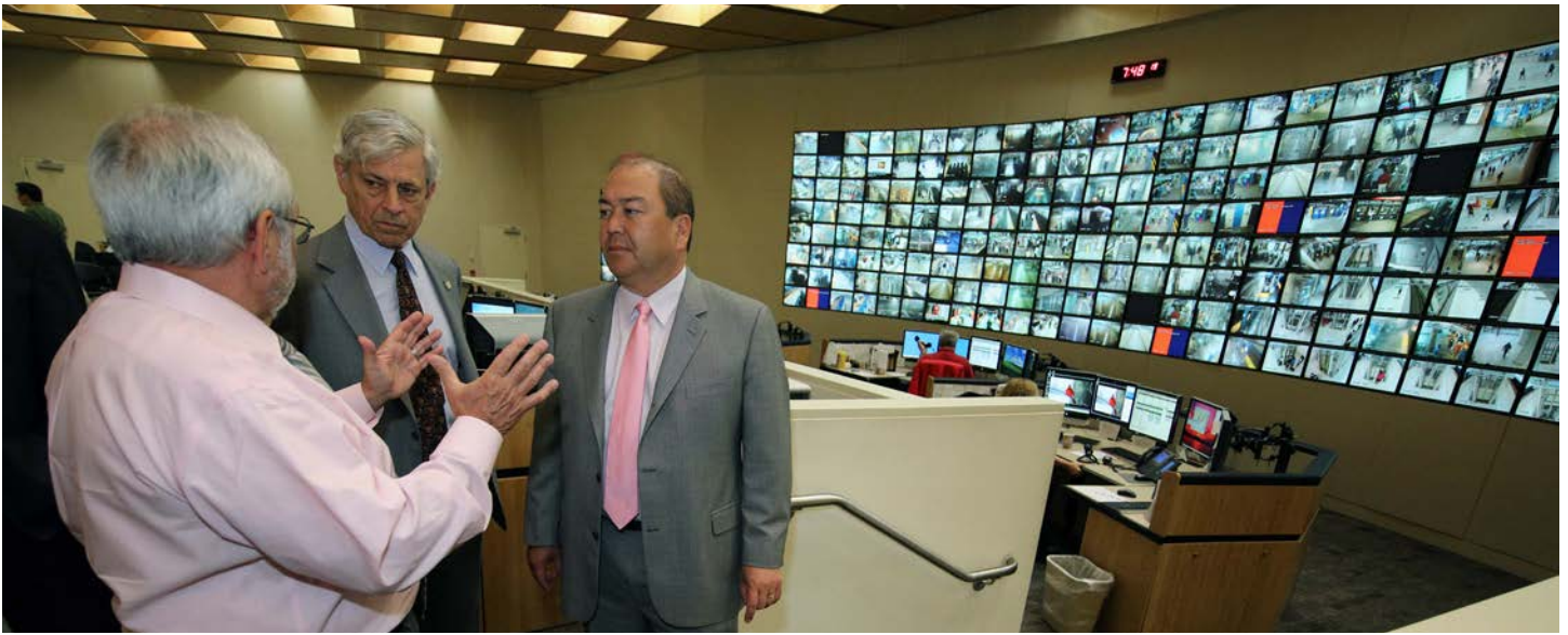
Chairman O'Toole and Executive Director Cotton get an overview of the PATH Train Control Center in Jersey City, NJ by Mike Marino, Director Rail Transit/General Manager PATH.
